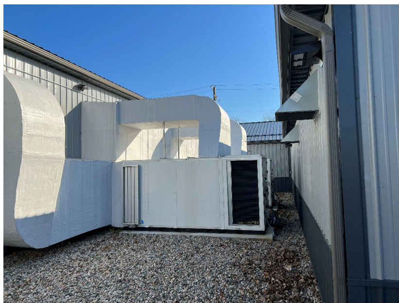
Figure 14. Air 2 O units supplying Flower Room
