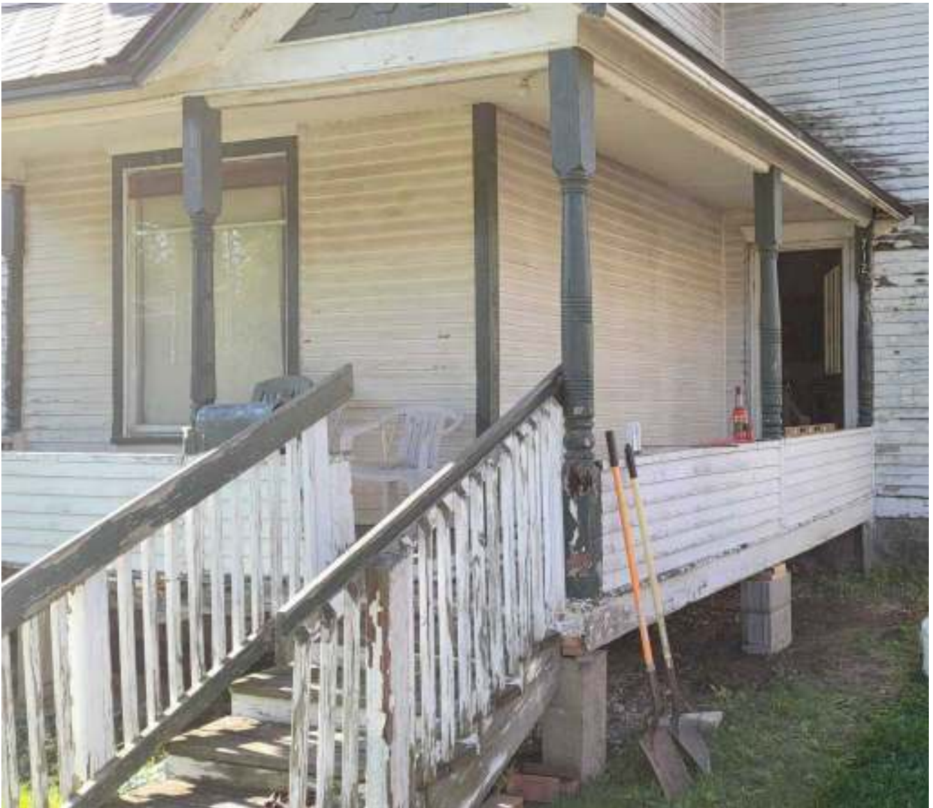
Picture 3: Rot on the southeast corner column
