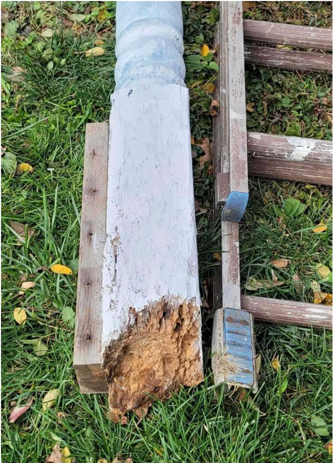
Picture 2: Rot on southwest corner column
