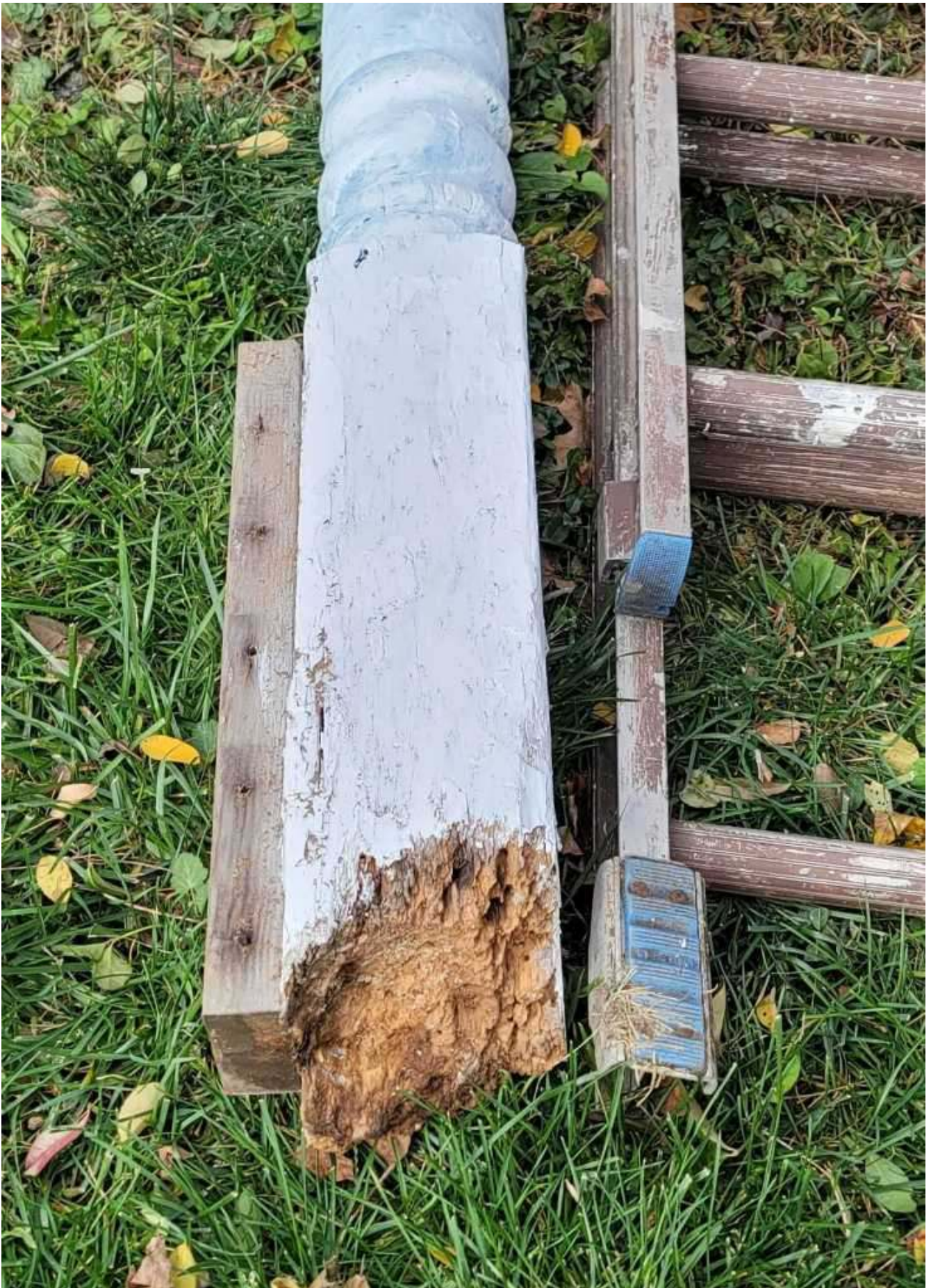
Picture 2: Rot on southwest corner column
