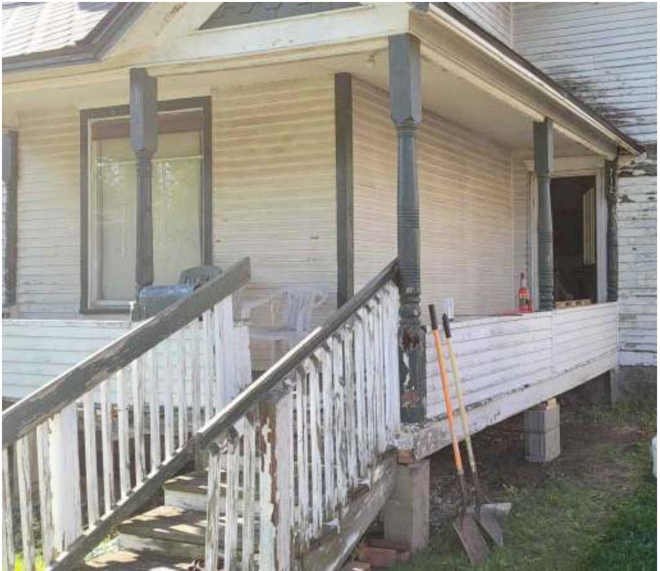
Picture 3: Rot on the southeast corner column
