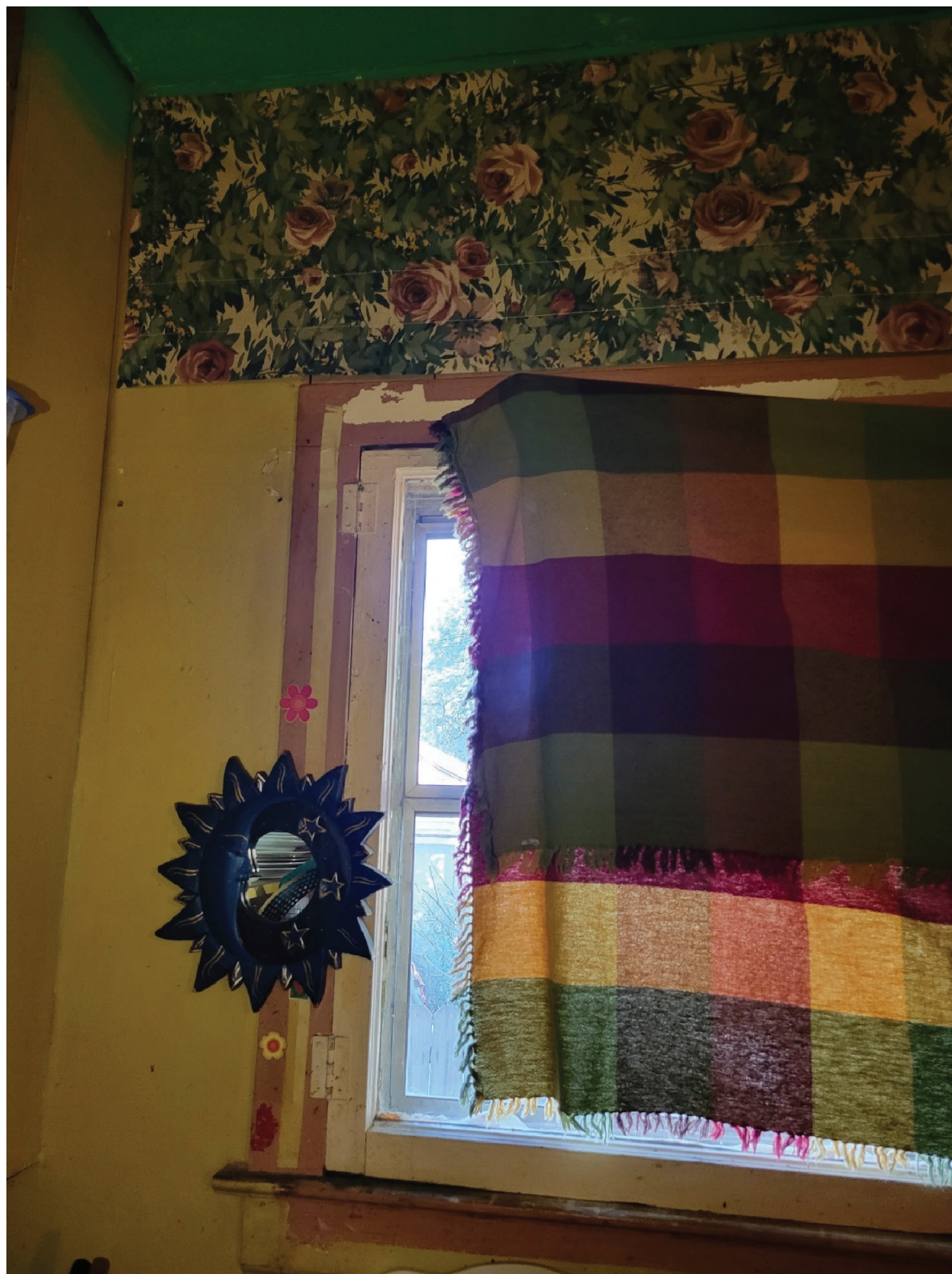
Kitchen window: Broken screen w/ tape holding pane together. Sash lead-based paint.
