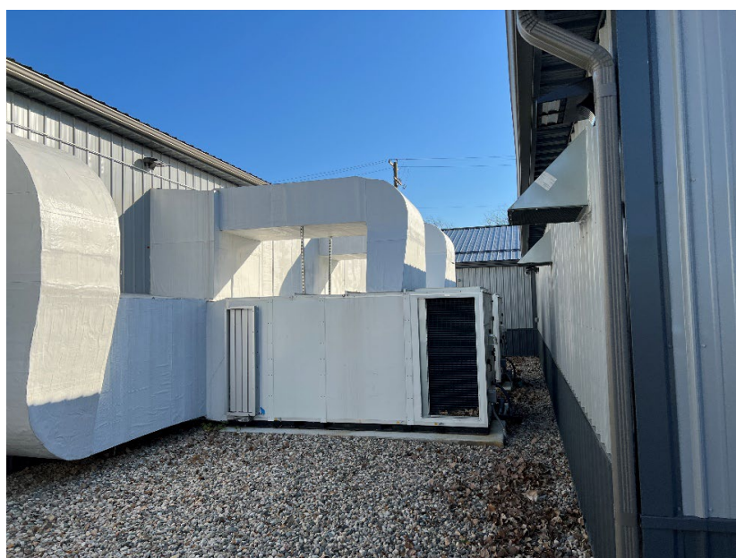
Figure 14. Air 2 O units supplying Flower Room
