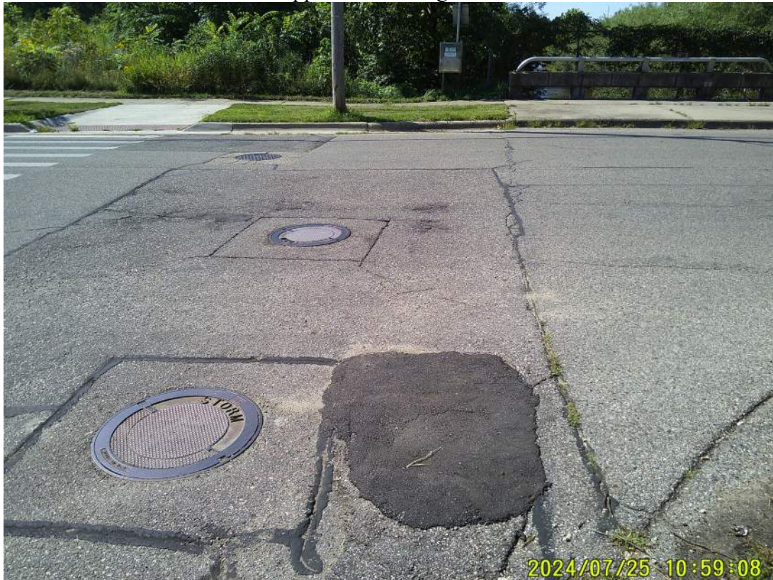
East Approach Condition
