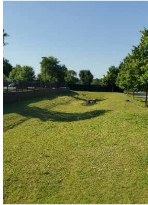
Detention basin at QT #1030, used to detain and slowly release runoff to capture sediment before it enters the stormwater system
