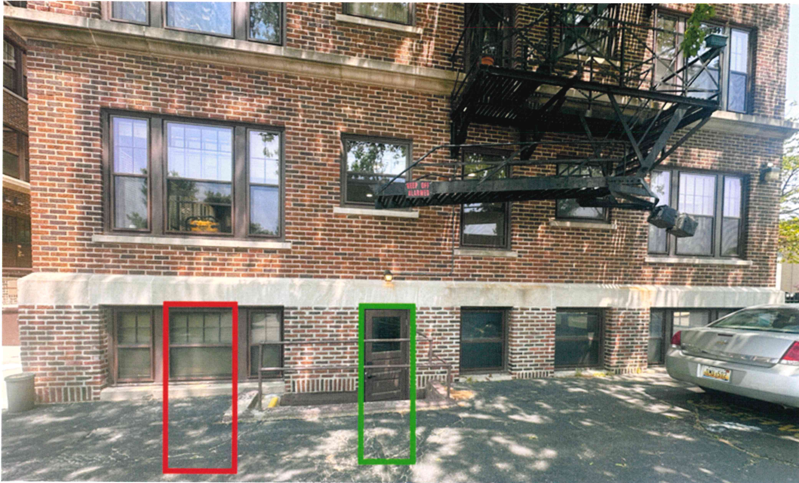
EXISTING ELEVATION OF SOUTH EXTERIOR WALL – LOCATION OF PROPOSED HANDICAP RAMP – NEW DOOR OPENING TO REPLACE EXISTING WINDOW (RED); EXISTING DOOR TO BE INFILLED WITH MATCHING WINDOW, BRICK VENEER, AND CAST STONE SILL
