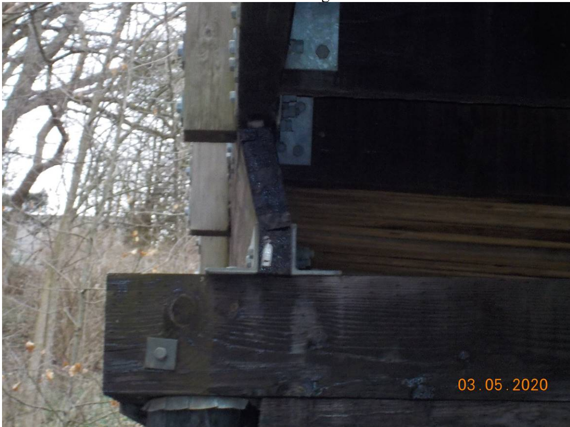
Distortion of north girder, center span under north sidewalk
