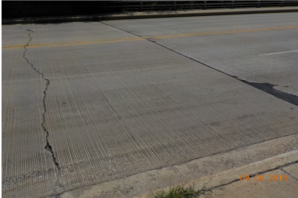
East Approach slab cracked
