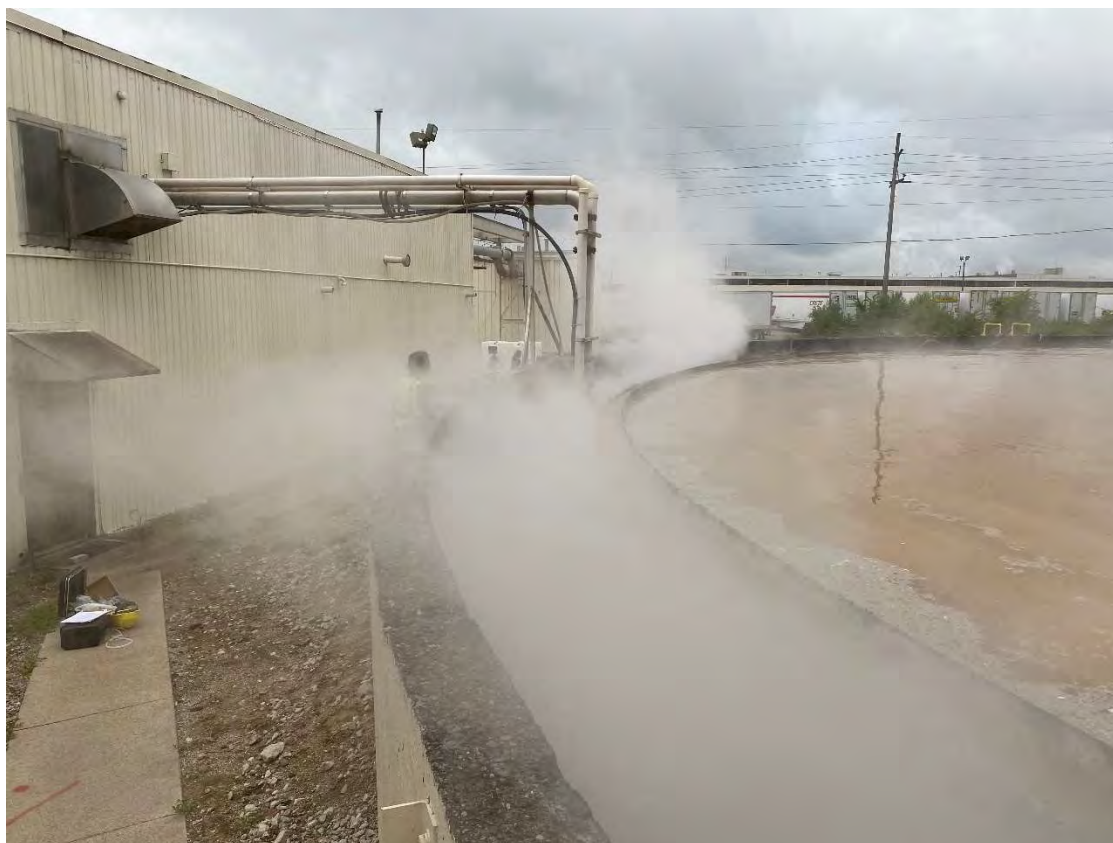
Sludge Drum Filter Outlet
